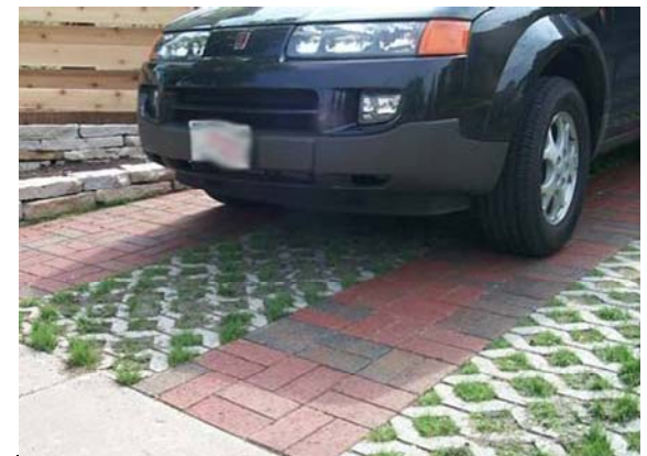
Permeable pavers in parking areas allow water to soak through; minimizing runoff.
